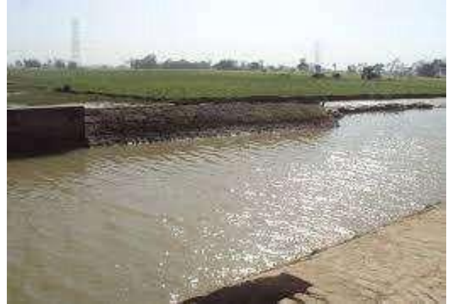
(a) Photo of barrage on Sone River at Indrapuri. The Eastern Canal System from barrage provides irrigation water in parts of western South Bihar Plains
